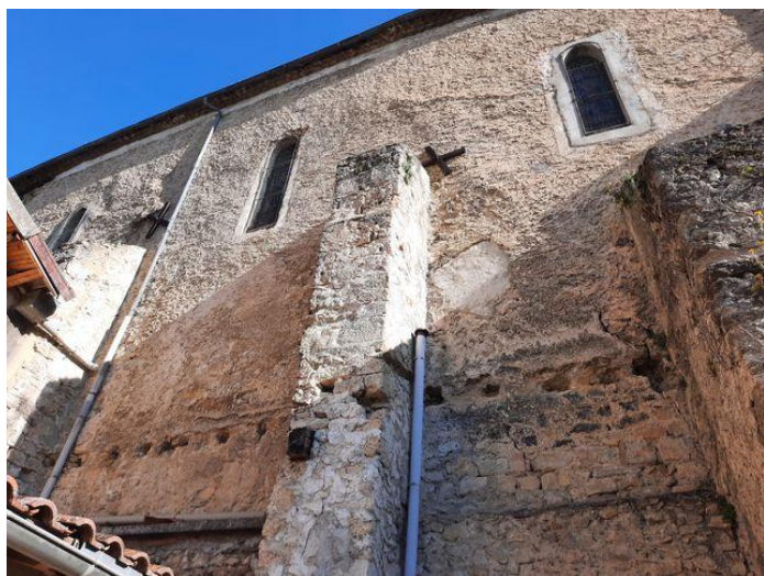
Fissuration de contrefort
